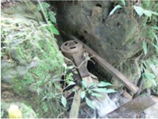
Mini-hydro installation in waterfall
