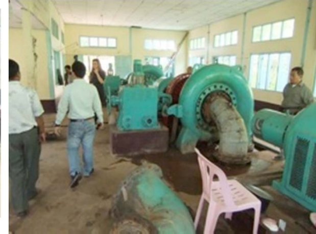
Hydropower Facility in Kengtung
