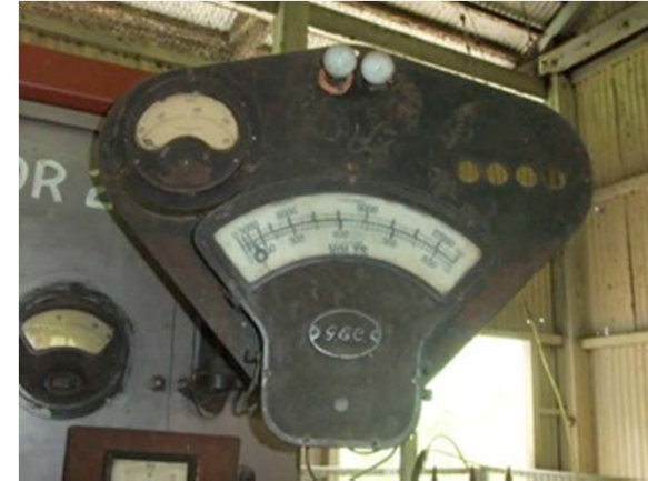
Hydro facility w/ equipment dating back to 1932
